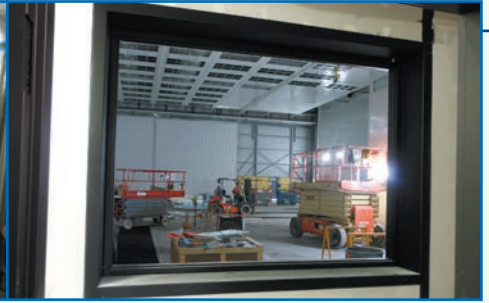
February 27, 2012 - Window into the down-draft bay.
